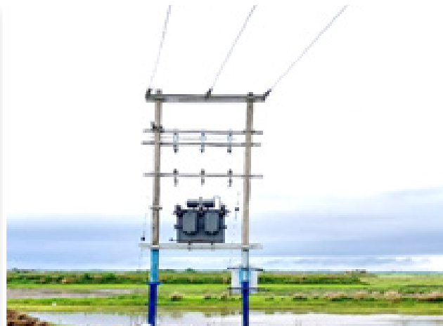
63 kva electricity connection
