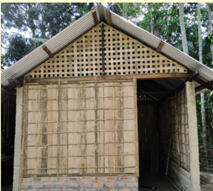
Construction of Eri Rearing House by Smt. Tutumoni Phukan at Lahdoigarh in Jorhat District.
